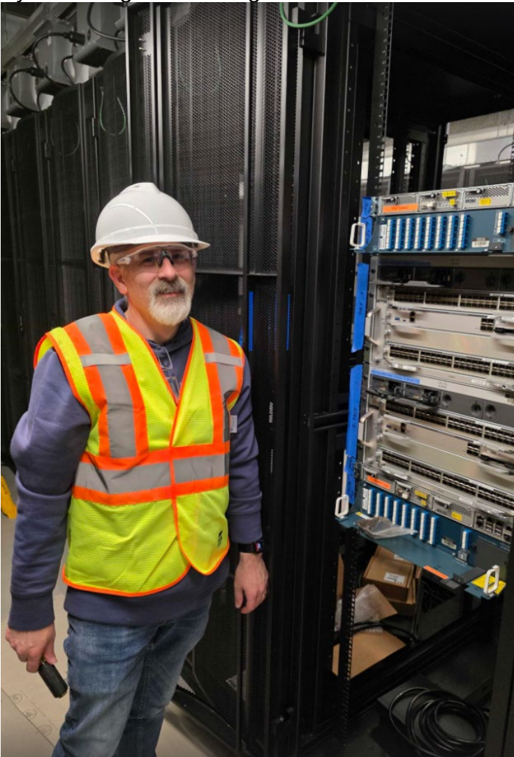
Systems Engineer racking servers in the data center.
