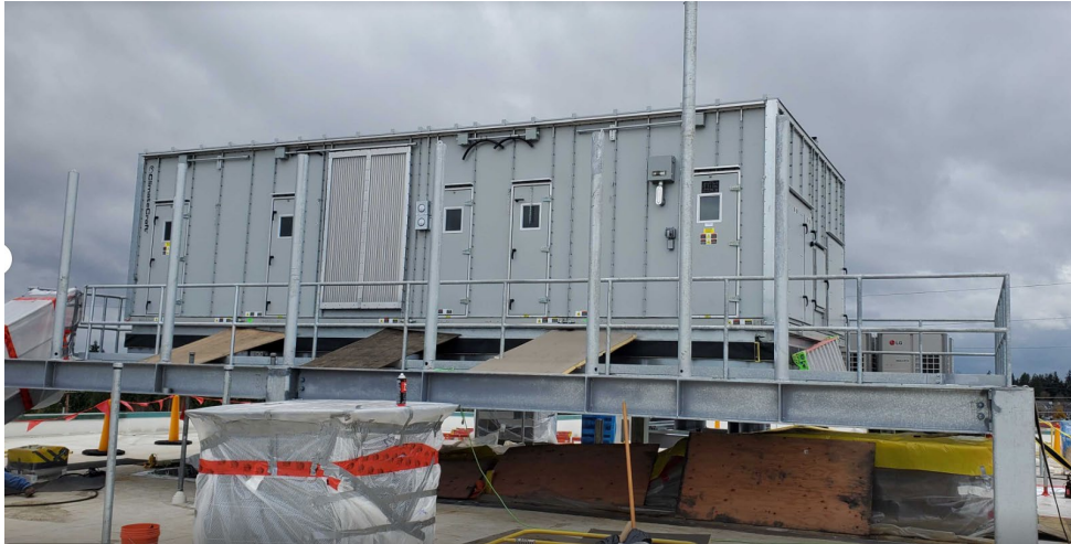
Building B Rooftop HVAC
