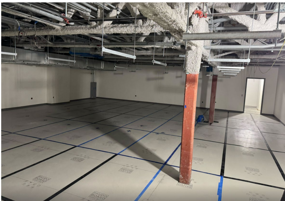
Server Room (before CRAC installation)
