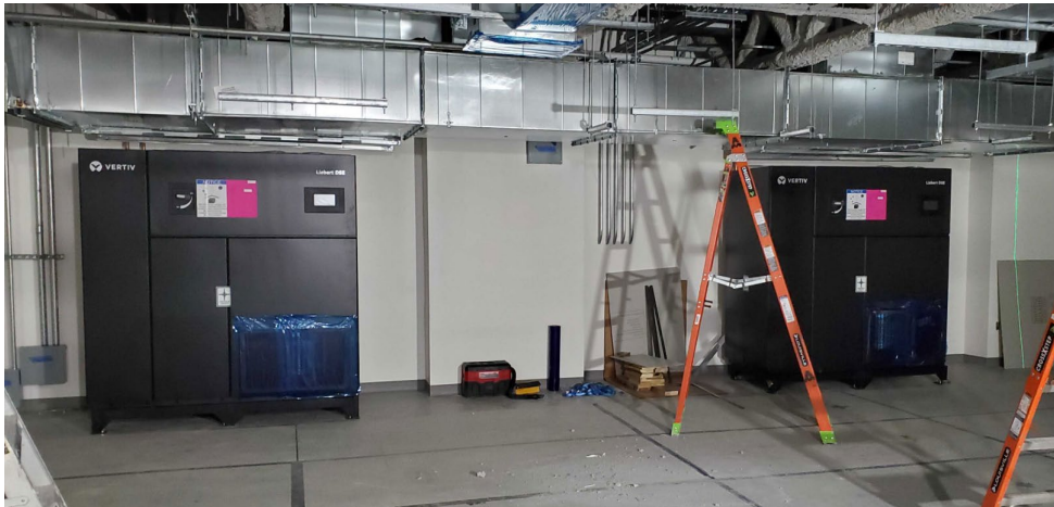
Server Room Redundant CRACs (Computer Room Airconditioning)
