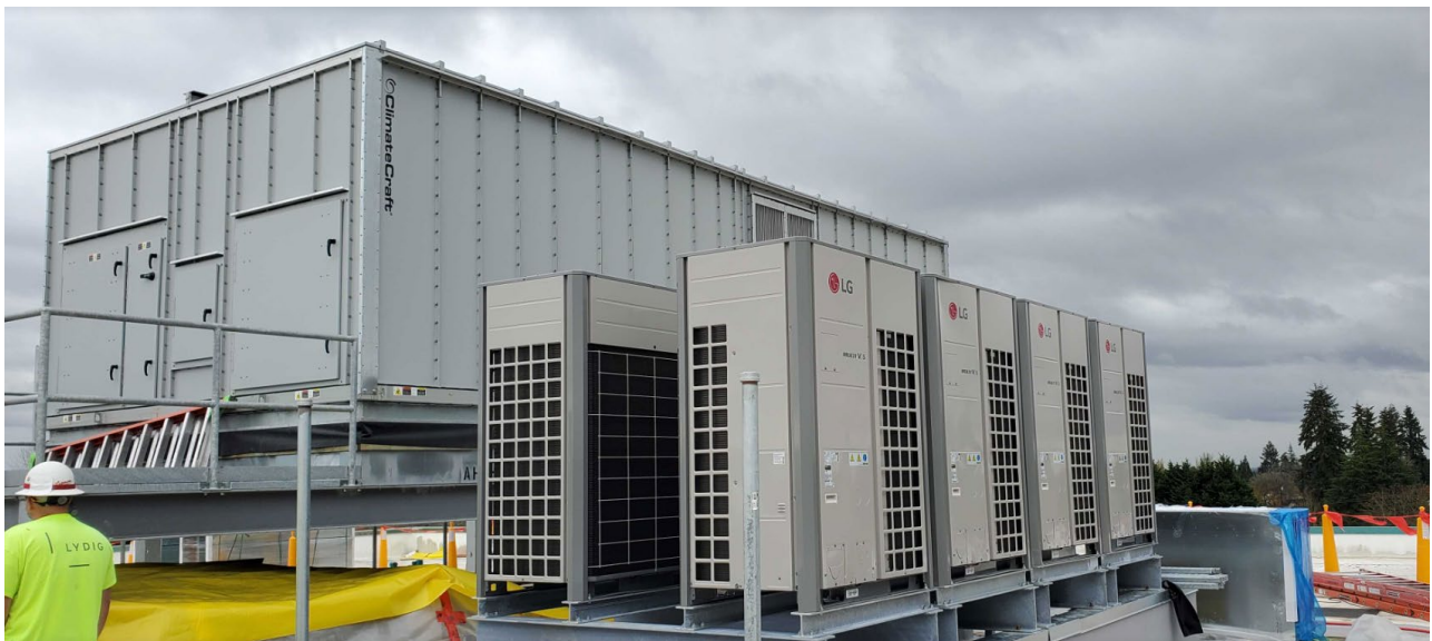
Building B's Rooftop HVAC
