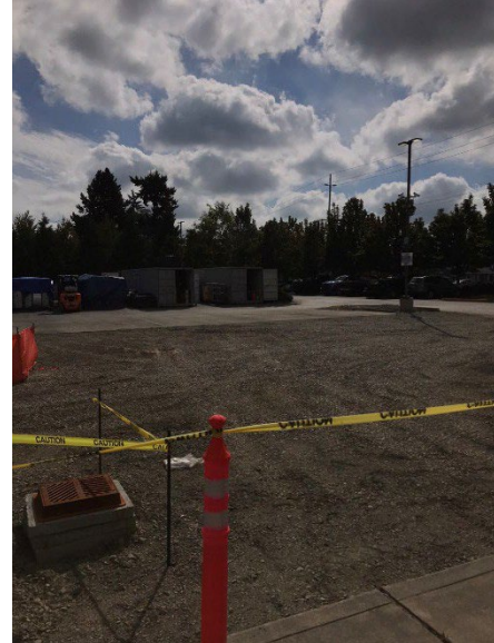
Storm water Retention Tank Covered
