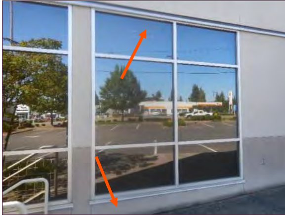
Photo 5.1.1.1-3: Typical head/floorline flashing clearance
