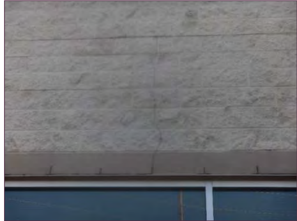
Photo 5.1.2.1-2: Crack in veneer/mortar, NW corner
