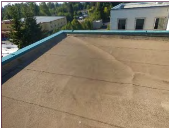
Photo 5.1.1.2-3: Roof membrane expansion
