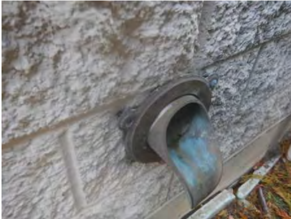
Photo 5.1.2.4-1: Unsealed penetration at scupper
