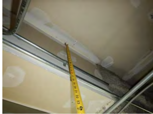
Photo 5.2.1.2-2: Concealed Glulam beam dropping 18 inches below 14-inch deep TJI floor framing
