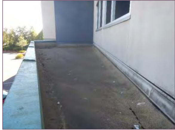
Photo 5.1.1.4-4: Canopy roof requires cleaning
