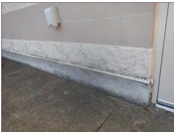
Photo 5.1.2.1-5: Base wall flashing, weeps blocked
