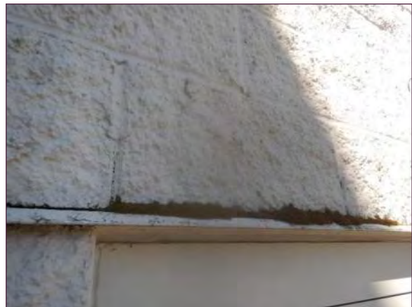
Photo 5.1.2.1-4: Weeps blocked, growth at flashing
