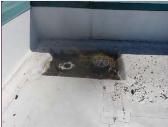
Photo 5.1.2.2-3: Debris/birds in sump area
