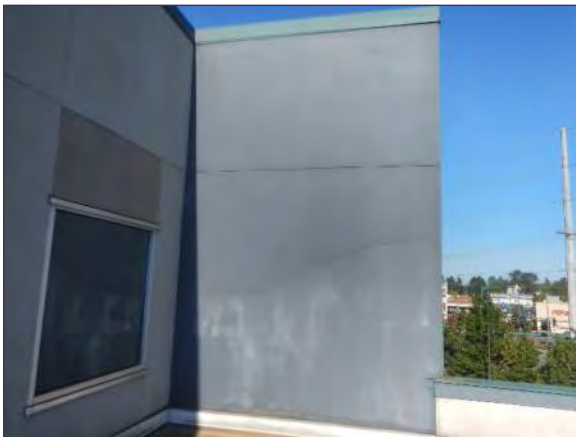
Photo 5.1.1.1-1: Stucco cracking, NW roof deck
