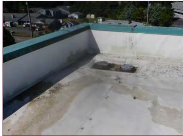
Photo 5.1.2.2-2: Staining, telegraphing fasteners
