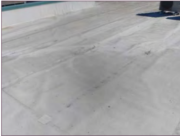
Photo 5.1.2.2-1: Telegraphing reinforcing/ fasteners
