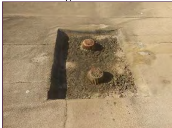
Photo 5.1.1.2-4: Sump area with debris SE corner
