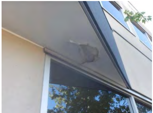
Photo 5.1.1.4-2: Soffit coating checking/peeling
