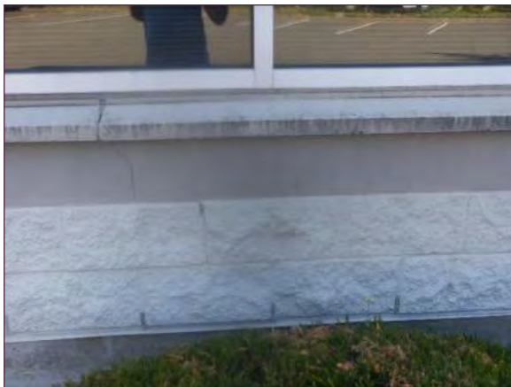
Photo 5.1.2.1-3: Crack in veneer/mortar, NW corner
