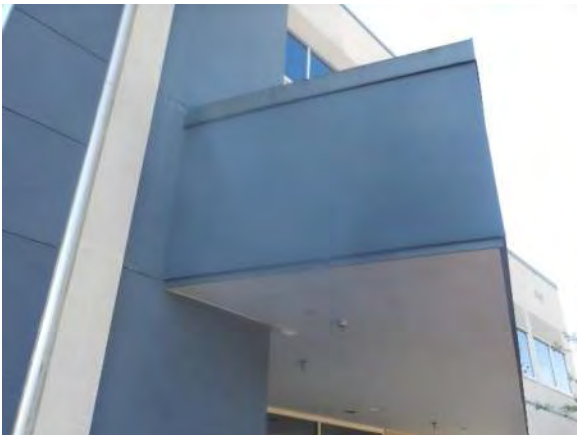
Photo 5.1.1.4-1: Soffit coating peeling (below drain)
