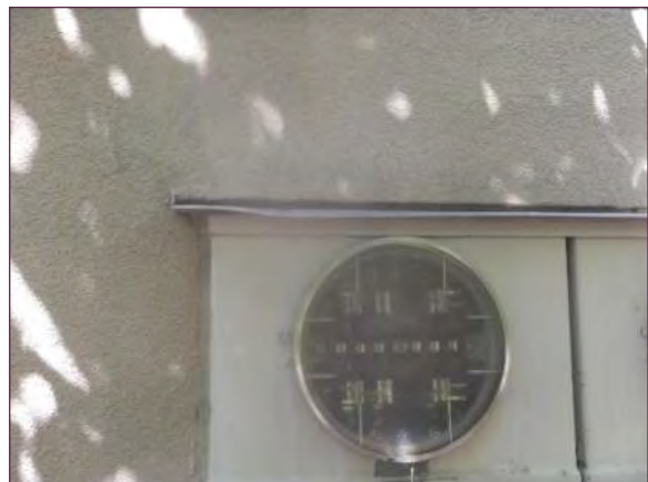
Photo 5.1.1.1-6: Meter boxes with flashing
