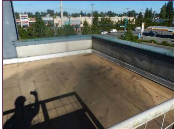
Photo 5.1.1.2-2: NW roof deck roof membrane, typical debris
