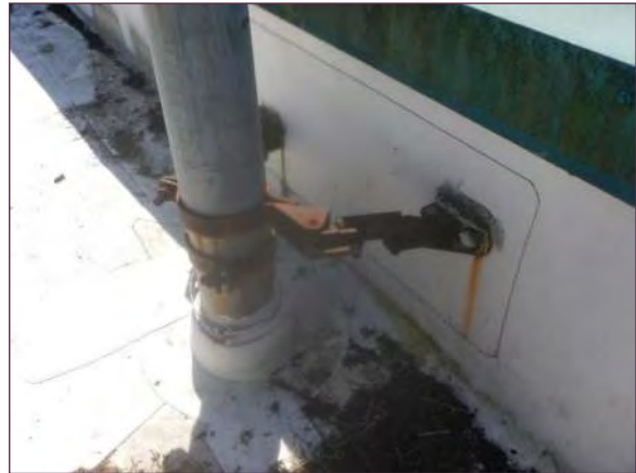
Photo 5.1.2.2-4: Vent stack support through membrane
